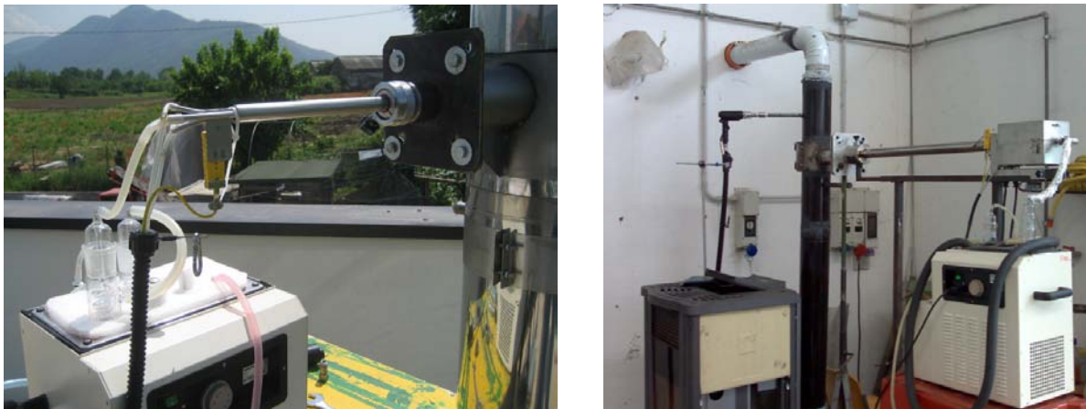
Figure 2. Ministack probe on boiler chimney (left) and pellet stove (right).
